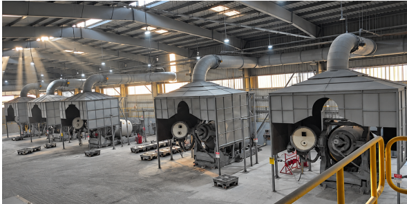
Image 2: PyroGenesis' Drosrite™ systems ready for use at Radian Oil & Gas Services' facility in Saudi Arabia.
