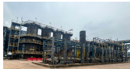
Image: PyroGenesis' Coke Oven Gas and Hydrogen Extraction System at Tata Steel, Kalinganagar, India.
