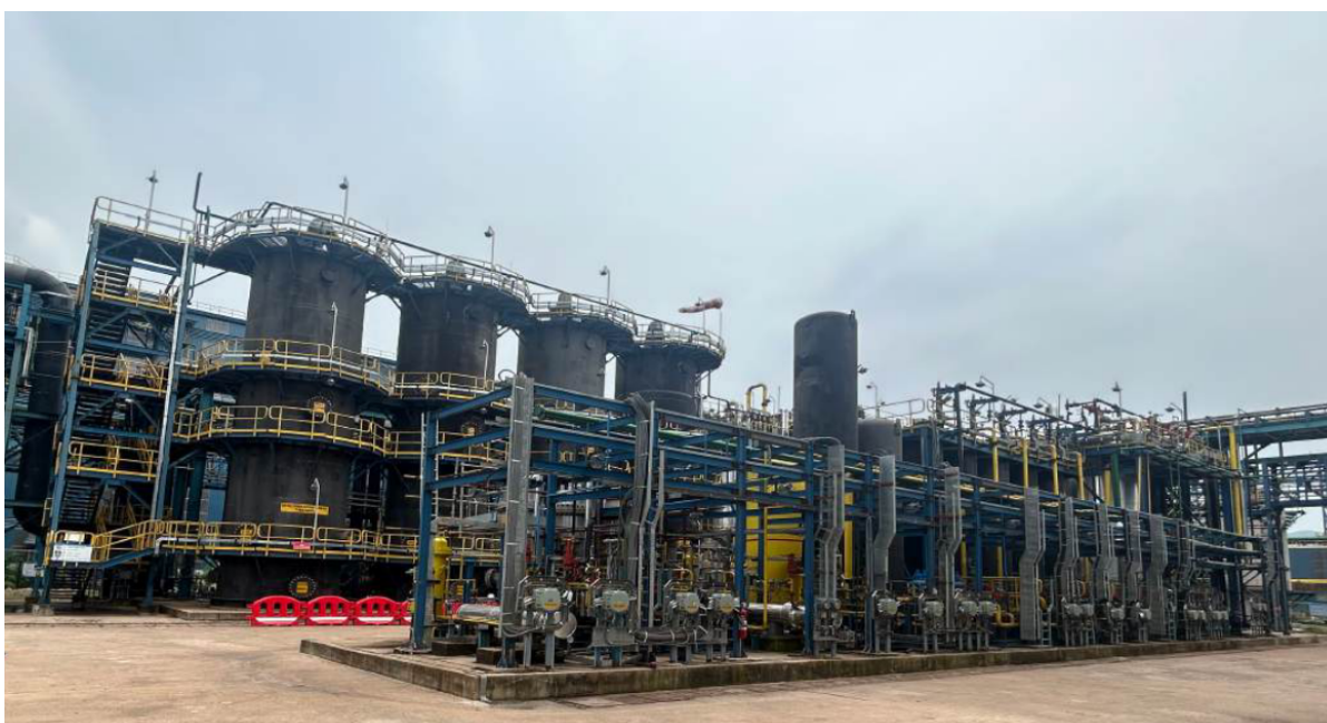
Image: PyroGenesis' Coke Oven Gas and Hydrogen Extraction System at Tata Steel, Kalinganagar, India
